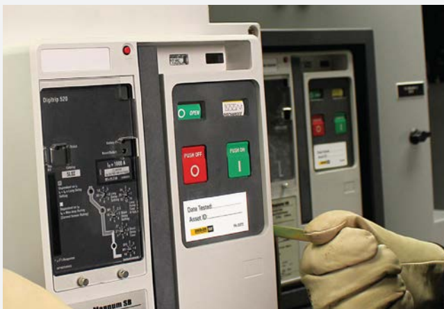
CIRCUIT BREAKER TESTING
