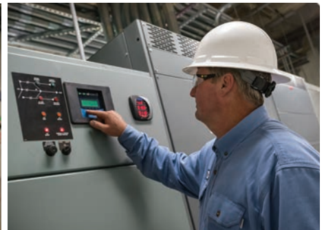
Automatic Transfer Switch Maintenance
