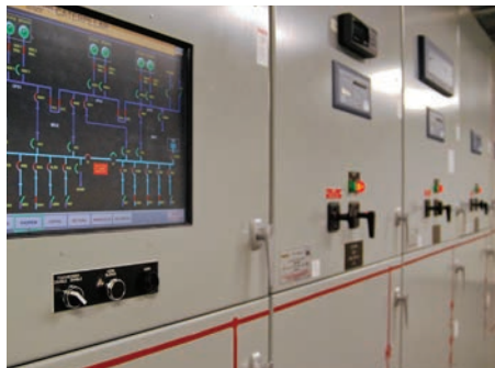
Switchgear Line Up
